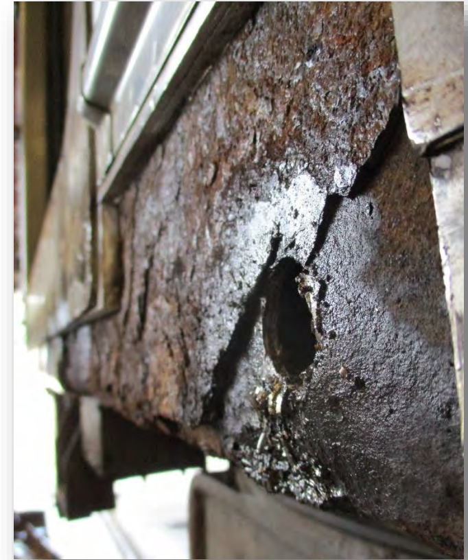
Corrosion Section Loss
