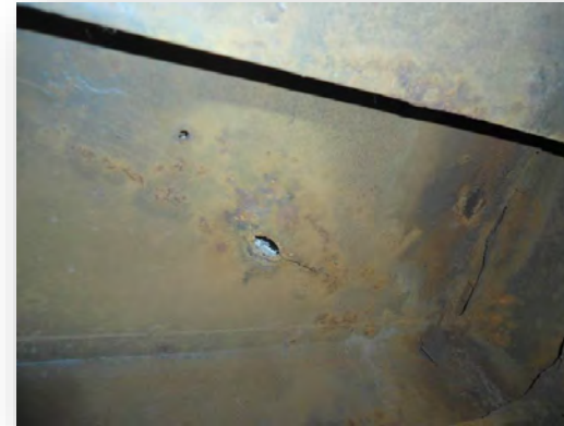
Corrosion Hole/Crack in Articulated Structure
